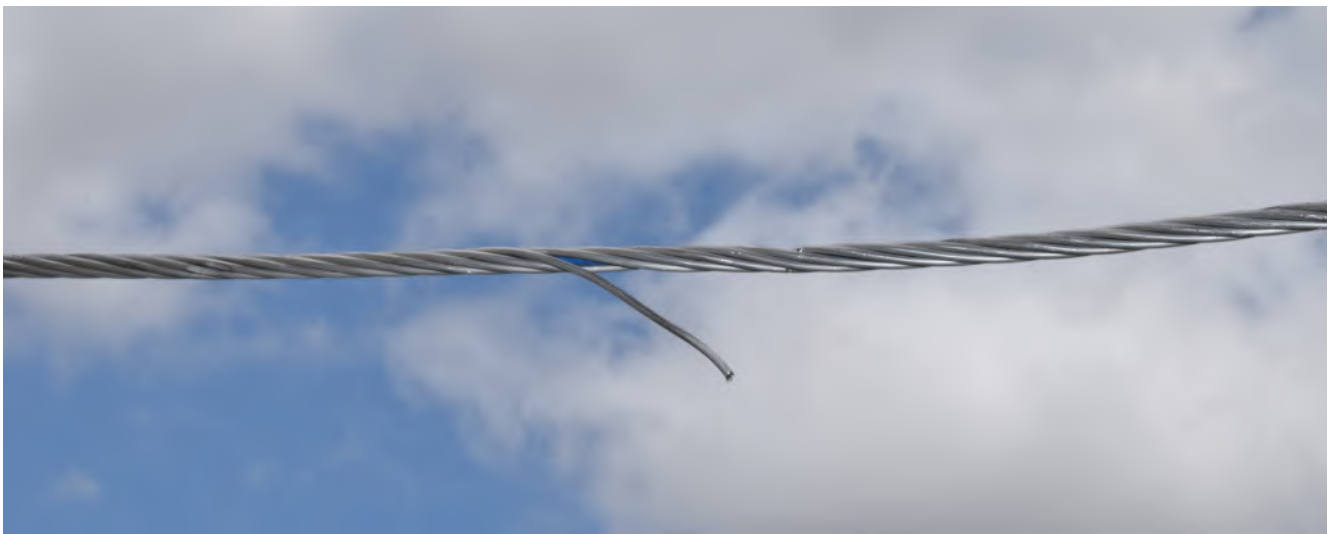
Figure 11 - Broken conductor strand clearly visible
