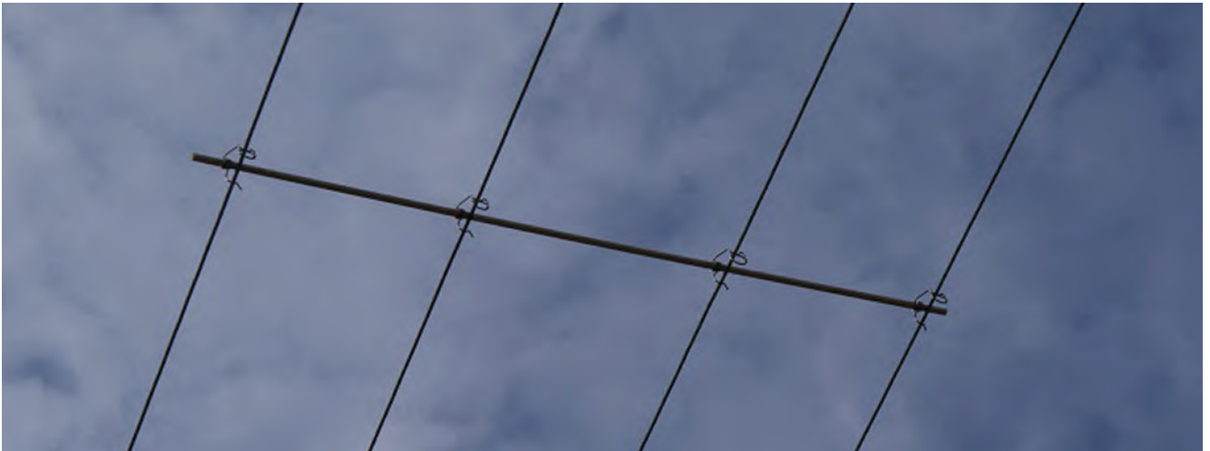
Figure 9 - Low voltage spreader in good condition
