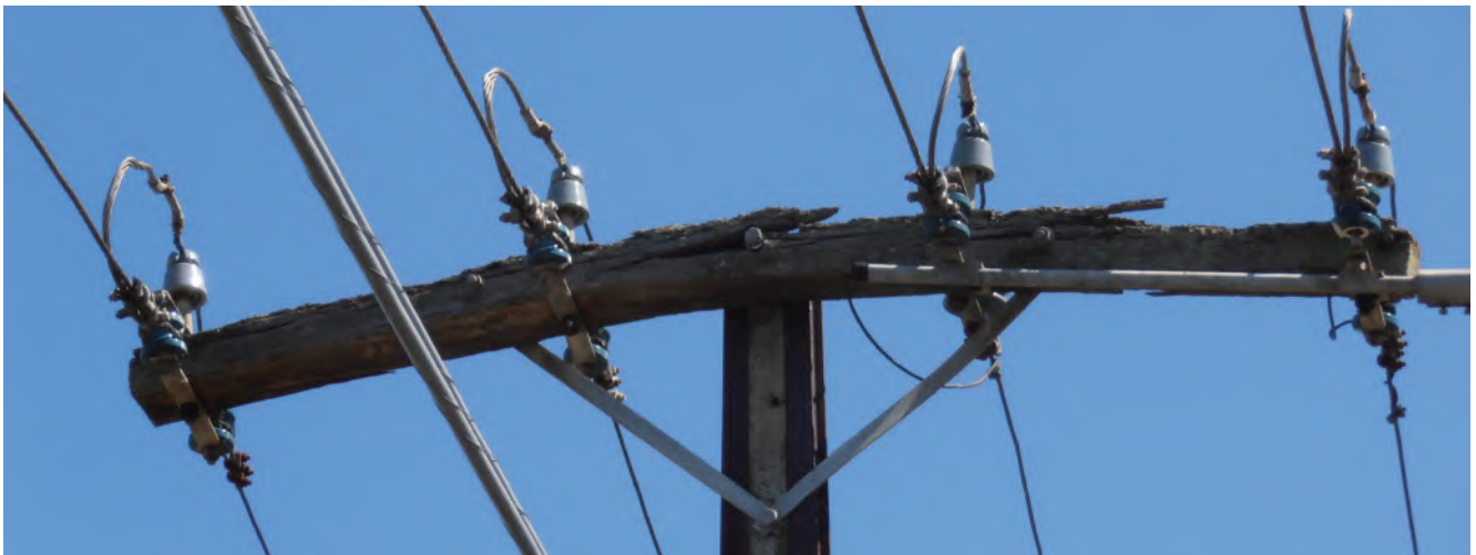
Figure 8 – A badly split low voltage crossarm
