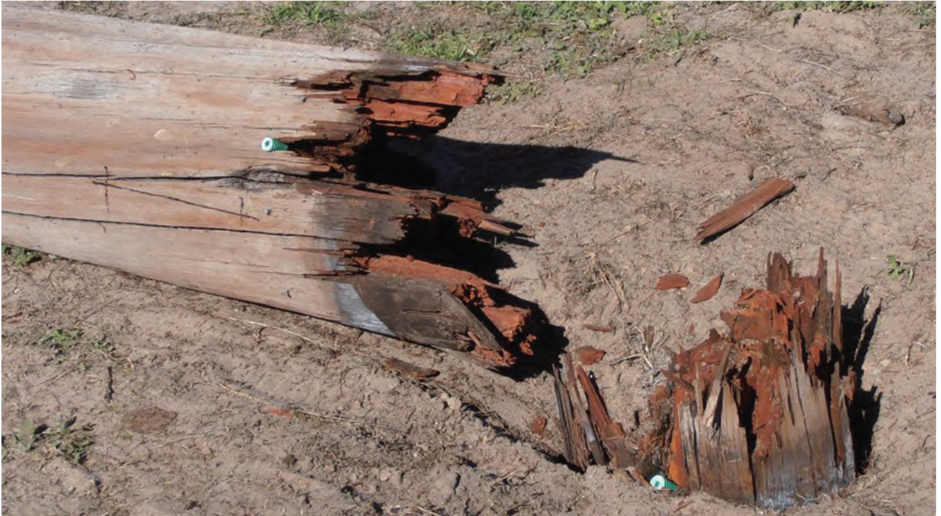
Figure 6 - Complete failure of Jarrah wood pole due to decay/rot at ground line
