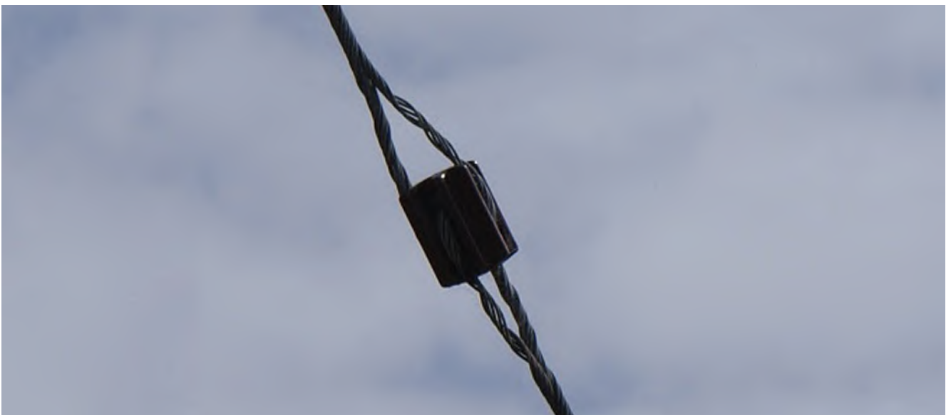
Figure 10 - Stay insulator correctly installed and in good condition
