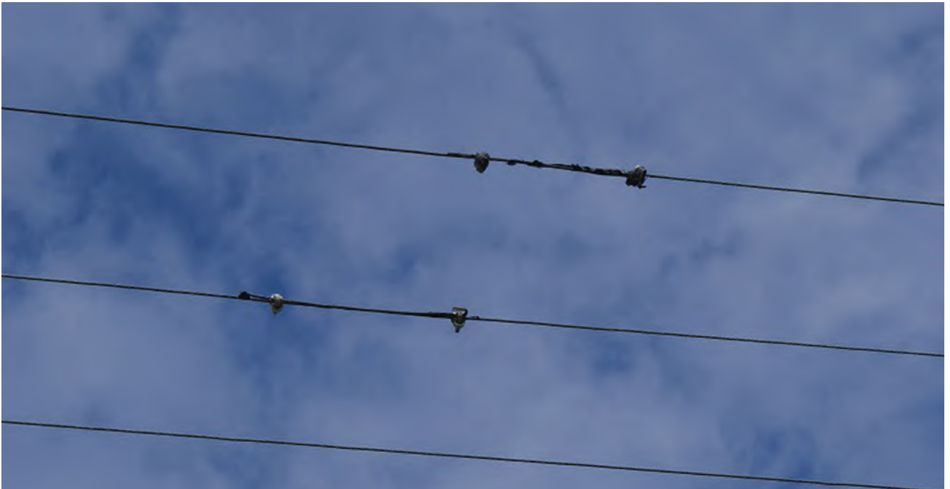
Figure 12 - Example of aged conductor joints and ongoing safety risk
